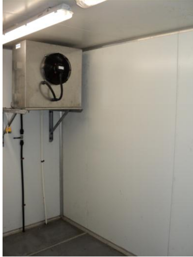
Plate 1 Interior of controlled temperature room
