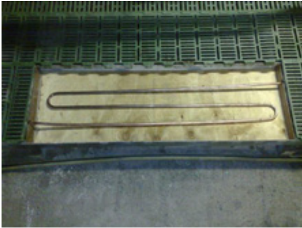
Figure 13. Typical copper pipe 'S' shaped section prior to pouring one of the concrete heating pads in the piggery farrowing sheds.
