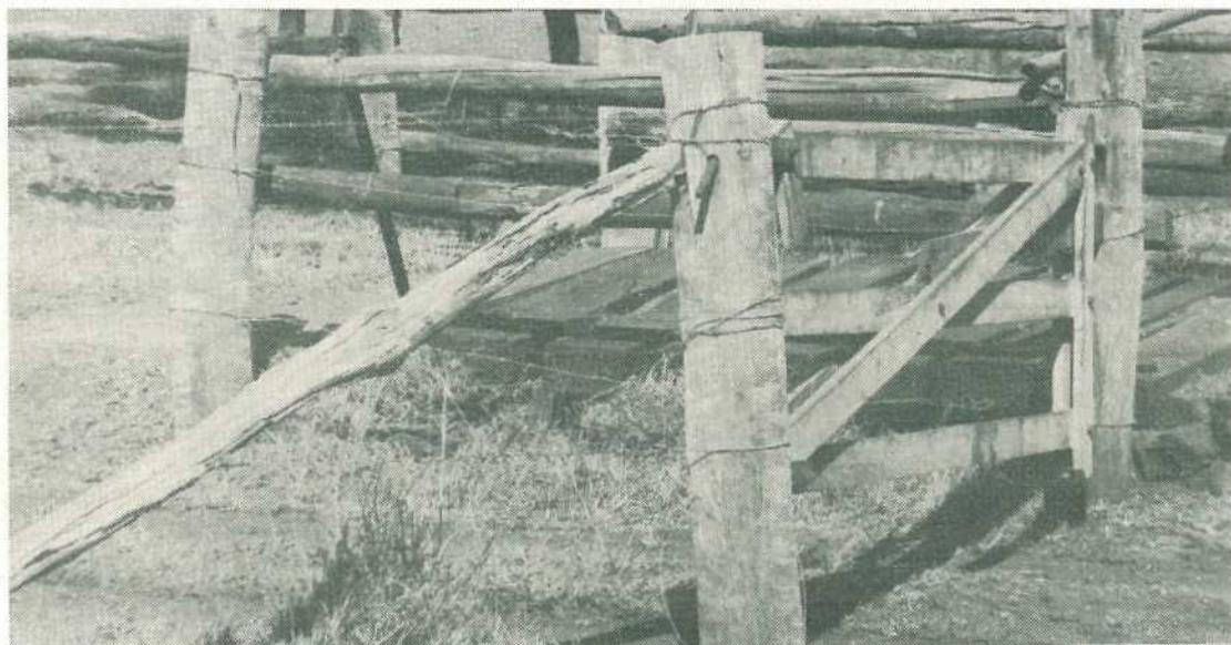
Wooden or steel gates can pull strainer posts over whether attached to an assembly or to the single strainer with a diagonal stay.
