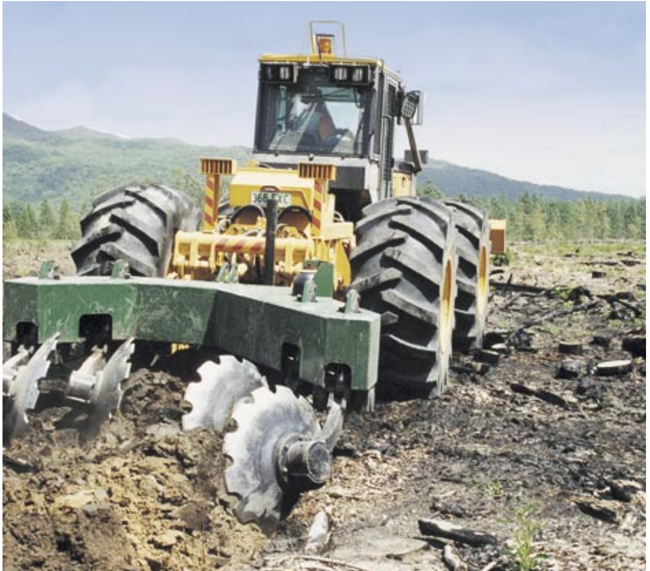
Site preparation for second rotation plantations, with a new $500,000 John Deere four-wheel-drive tractor, at Byfield in central Queensland.
