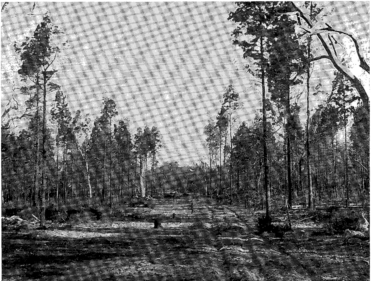
INTERNAL FIRELINE AND ACCESS TRACK IN CYPRESS PINE FOREST. 932 Miles of Fire Lines were constructed and 951 Miles maintained during the year.
