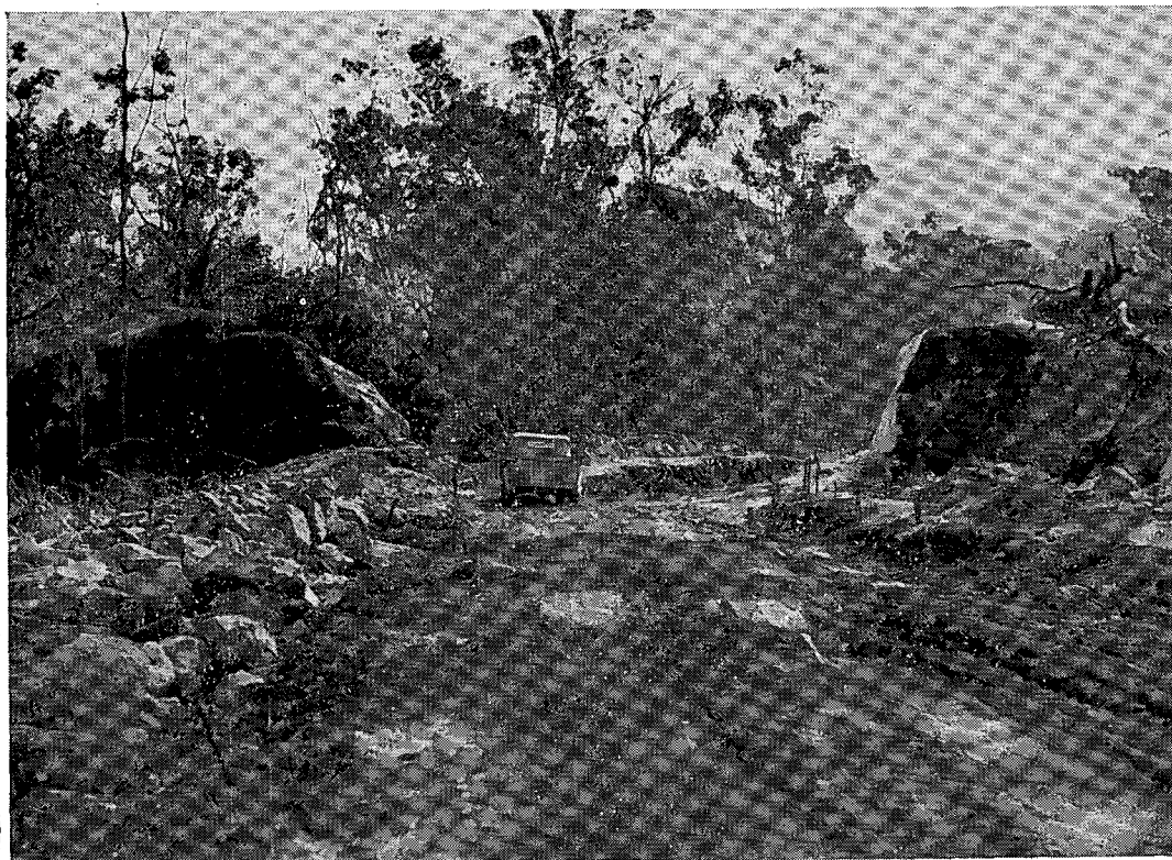
Kirrama Road Construction. In 1935-36 the sum of £64,467 was expended by Forestry Sub-Department in road construction, maintenance, and subsidies.
