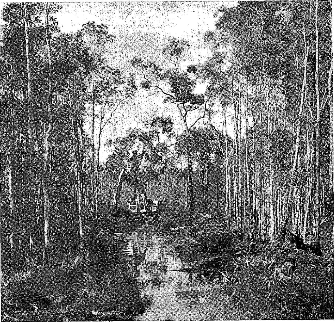
TRENCH DIGGER constructing Drainage Channel in preparation of area for planting. State Forest, 561, Bribe.
