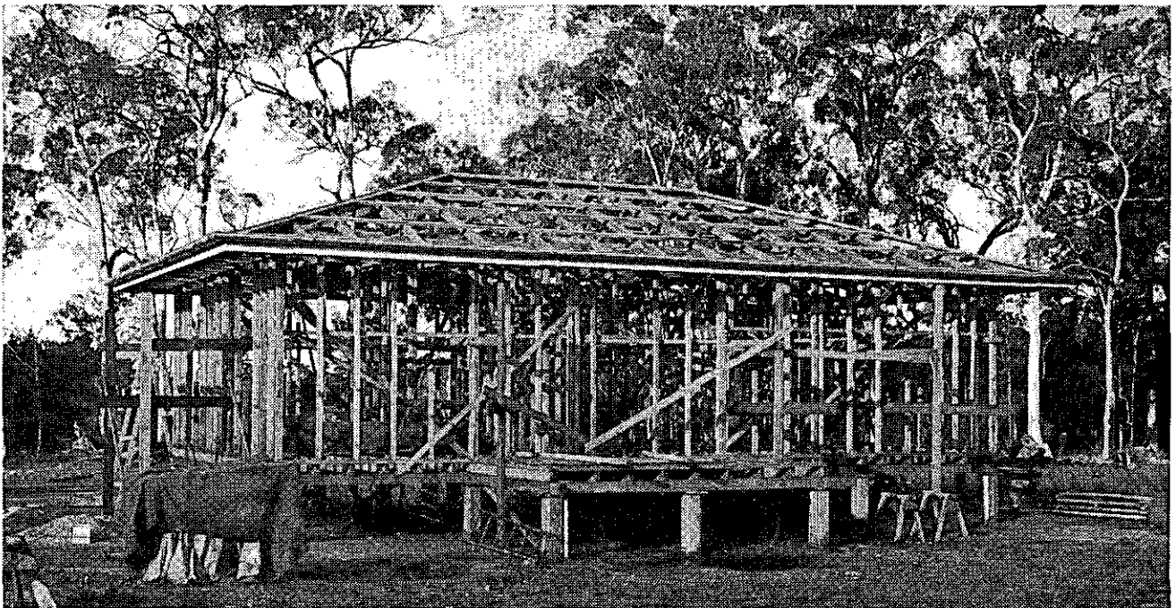
FORESTRY RESIDENCE, BEERBURRUM, UNDER CONSTRUCTION. Framing of unseasoned Slash Pine ( Pinus elliottii ) from Beerburrum plantations. Ground plates and roof battens of Scribbly Gum ( E. Micrantha ).
