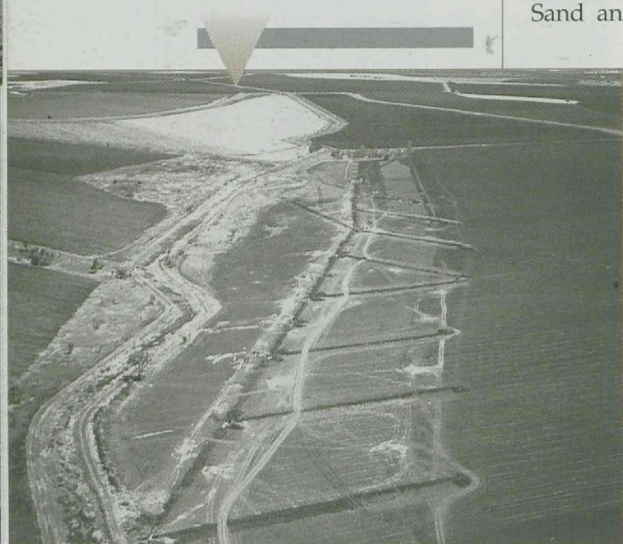
Drainage water flowing from a subsurface drainage network, Emerald Subsurface Drainage Project.
