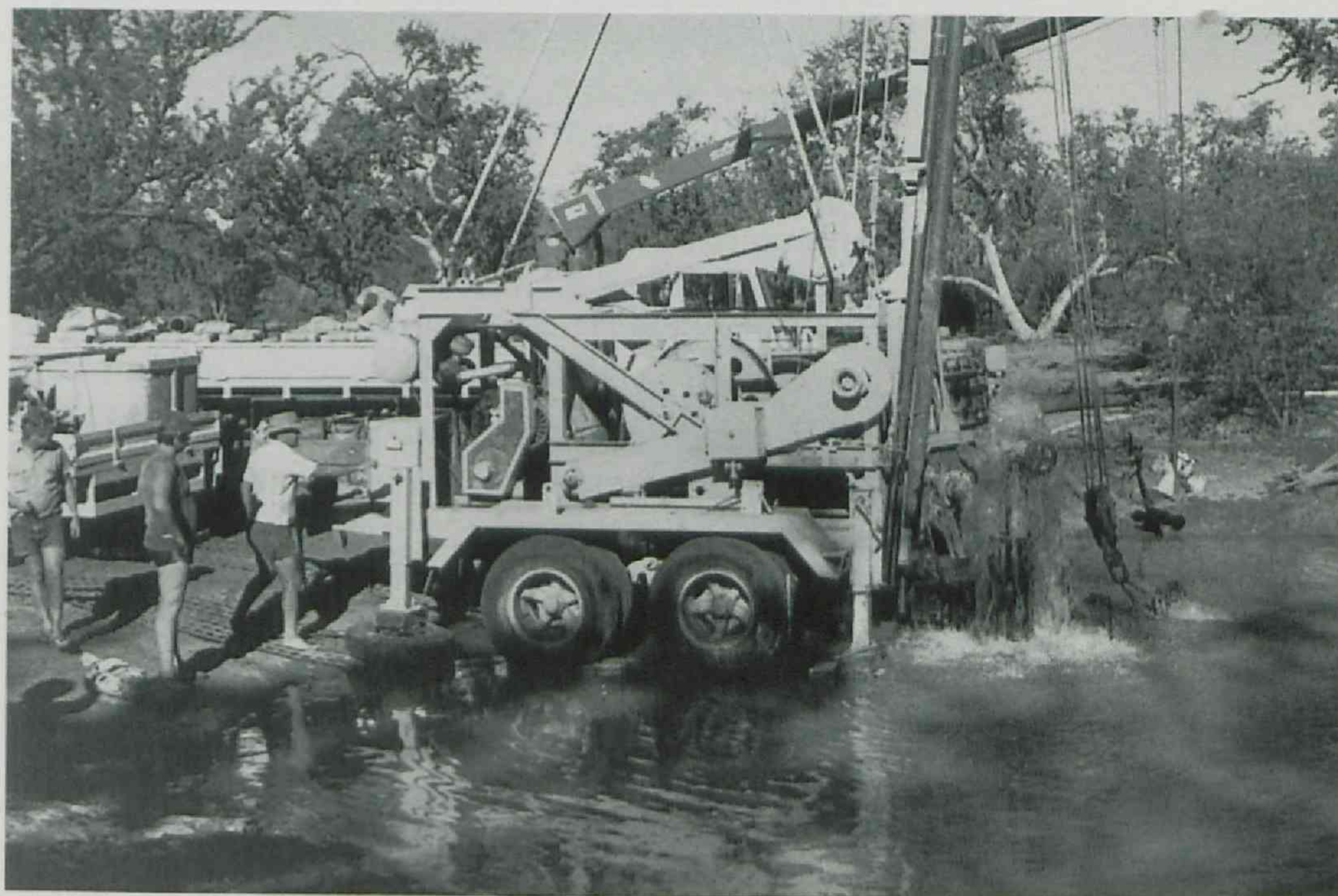
A Commission drilling rig reconditioning an uncontrolled bore near Richmond in western Queensland, as part of the Great Artesian Basin Rehabilitation Program.
