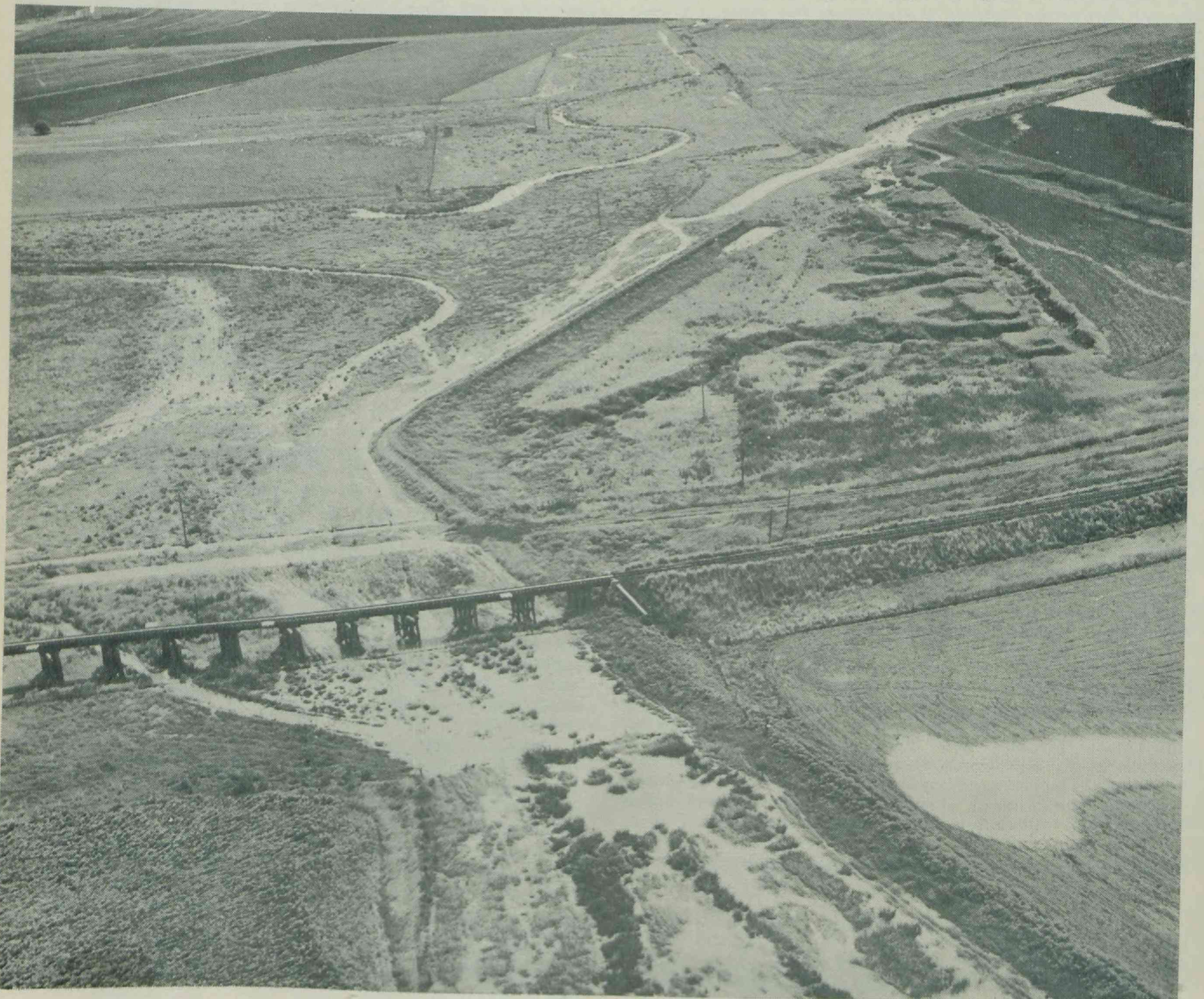
Successful completion of Stage 1 of the Emu Creek Stabilization Project—Cambooya Shire, Darling Downs.
