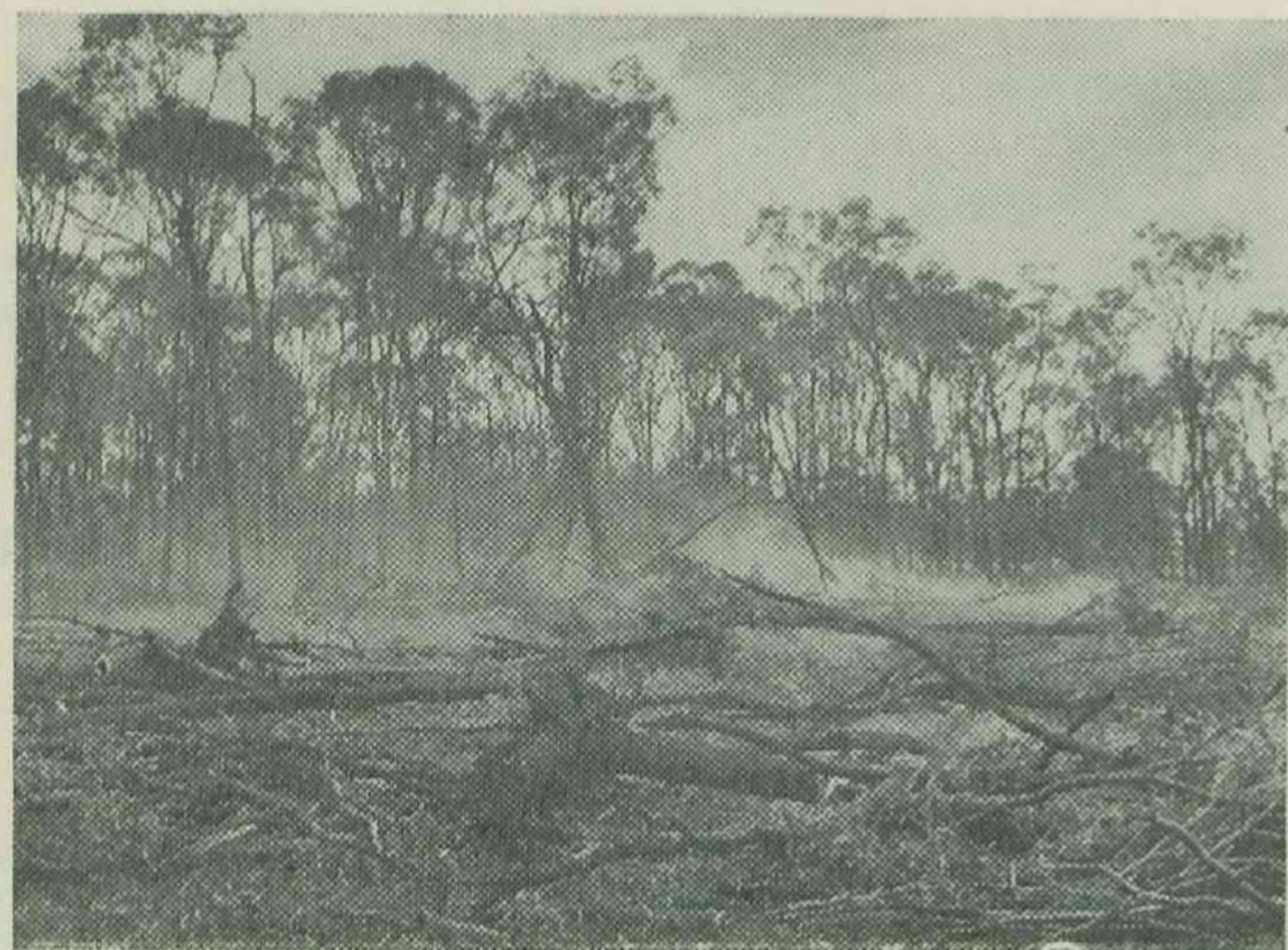
Departmental participation in land development schemes starts long before the clearing stage shown here.
