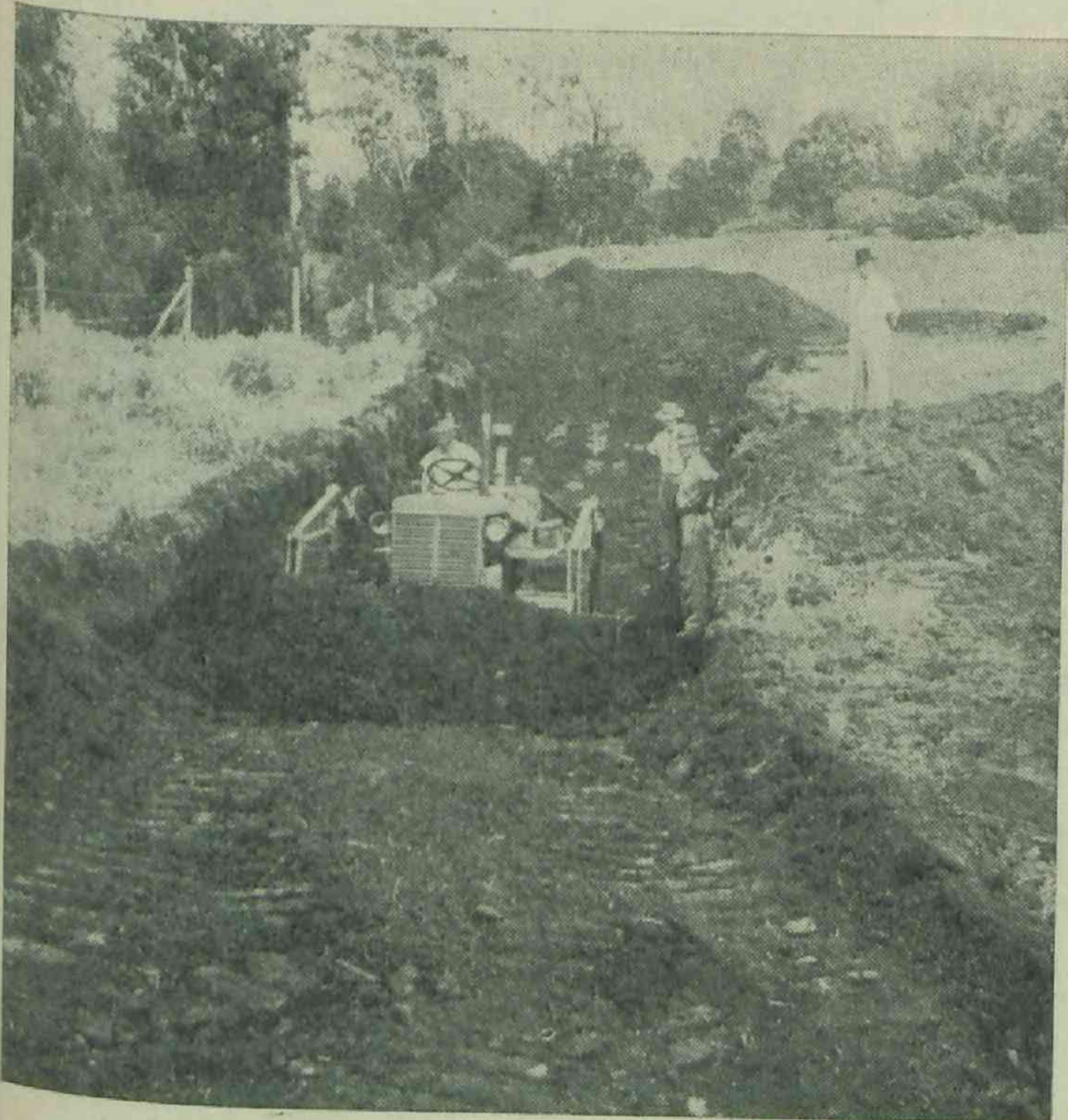
Plate 6.—Excavating a Trench Silo of a Capacity of About 140 Tons on a Central Queensland Property.
