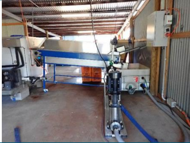
System view – HPW prior to hydrocooler
