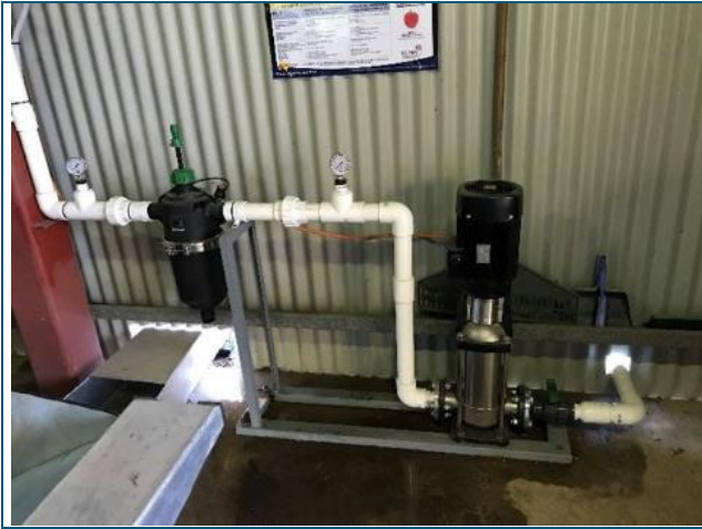
Pump and filter
