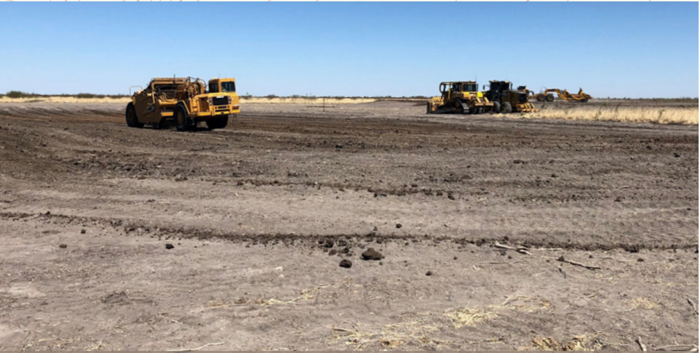
Photo 3. Constructing FRMs using the ideal range of earthmoving machinery including self-loading scrapers, bulldozer and a road grader. Photograph courtesy of A.A. Company Pty Ltd.
