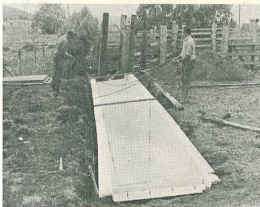
TOP. Turning the vat upright for the final lowering. BOTTOM. The vat in position.
