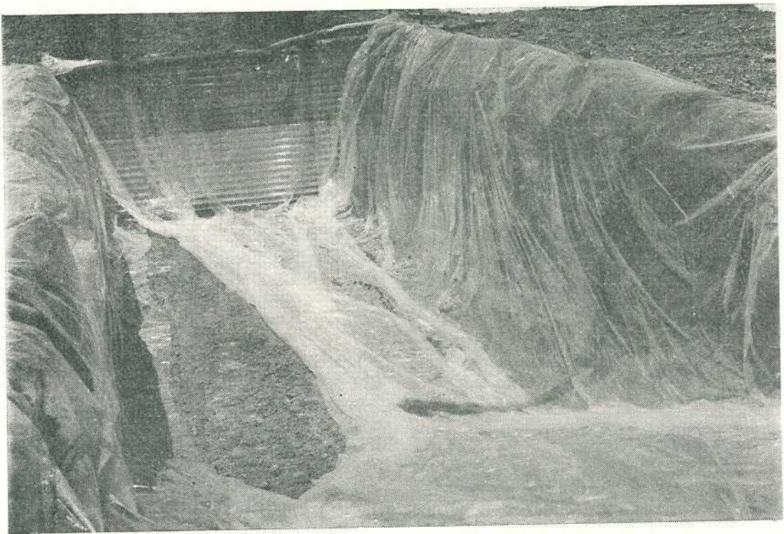
An underground pit in the Talwood district. Note the lining of polythene sheeting, prior to filling with grain.
