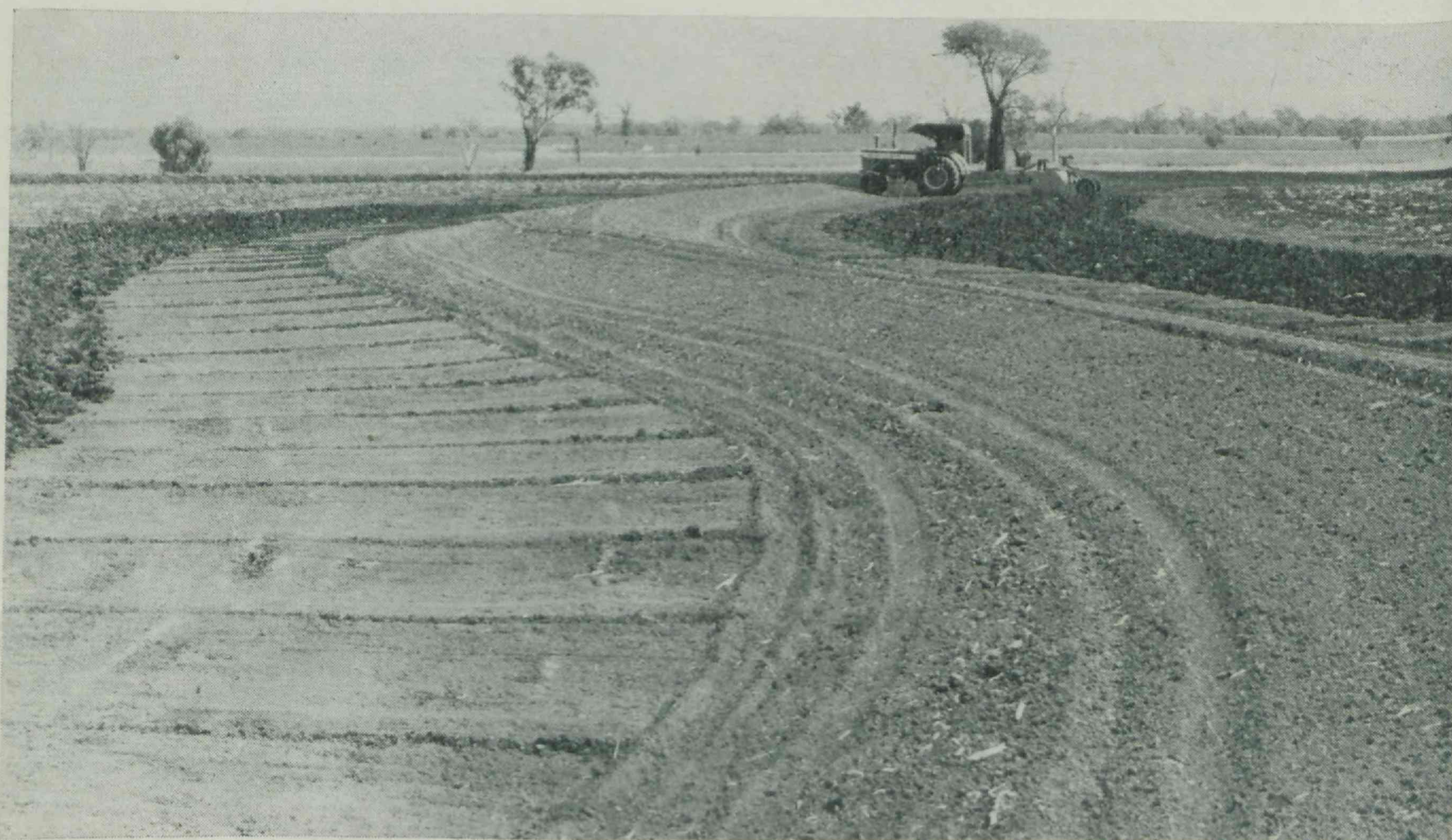
A farmer using a special tractor-drawn implement to build his own broad-based contour banks.
